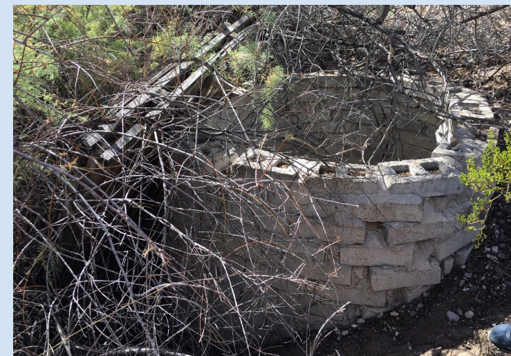
Hazardous condition at Summit Spring (a source shared with the BLM), pre-restoration
